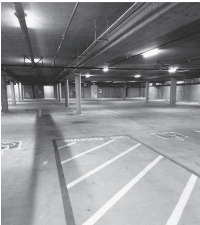
A view of the parking level, virtually complete. The only thing we plan to do there is to mark the pillars with reflective material.
