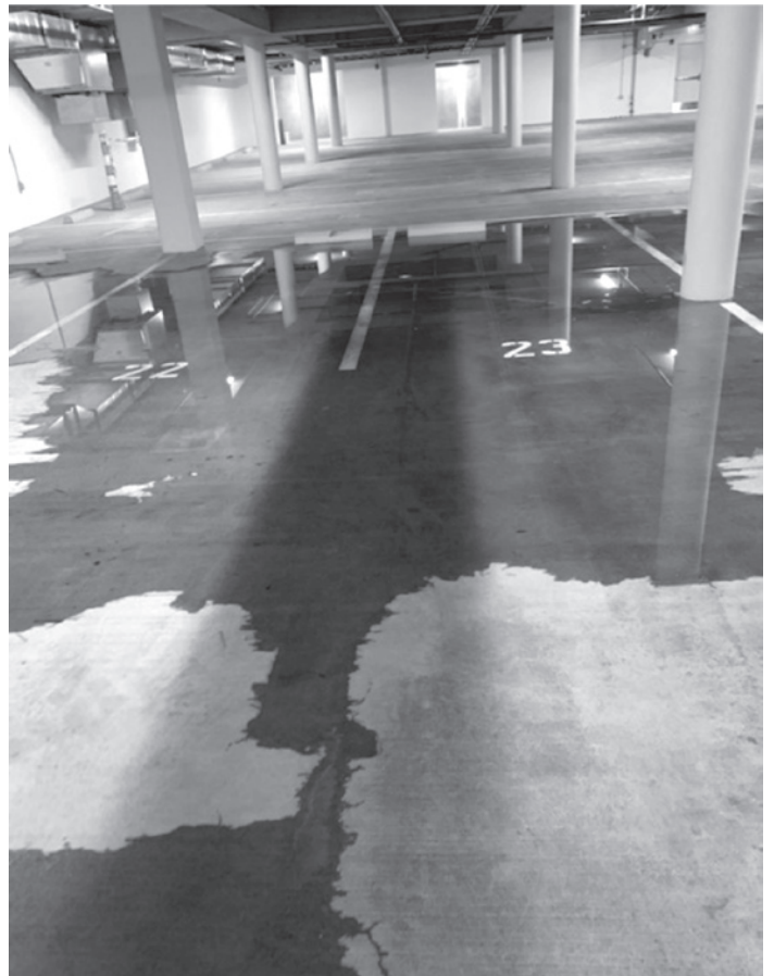
Water from above found its way into the garage.
