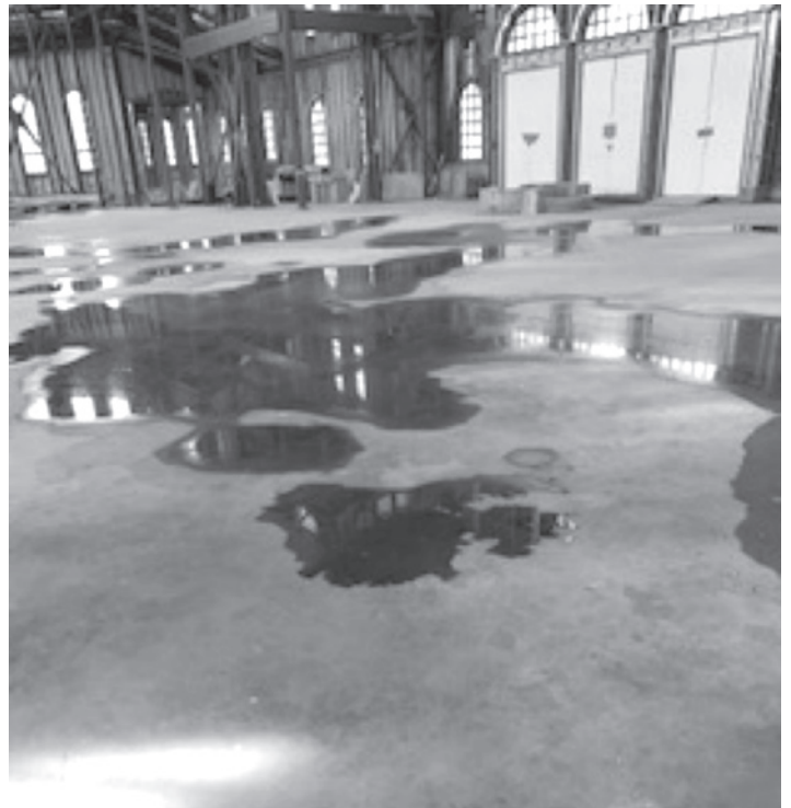
Overall view of the interior following the rains on December 7.
