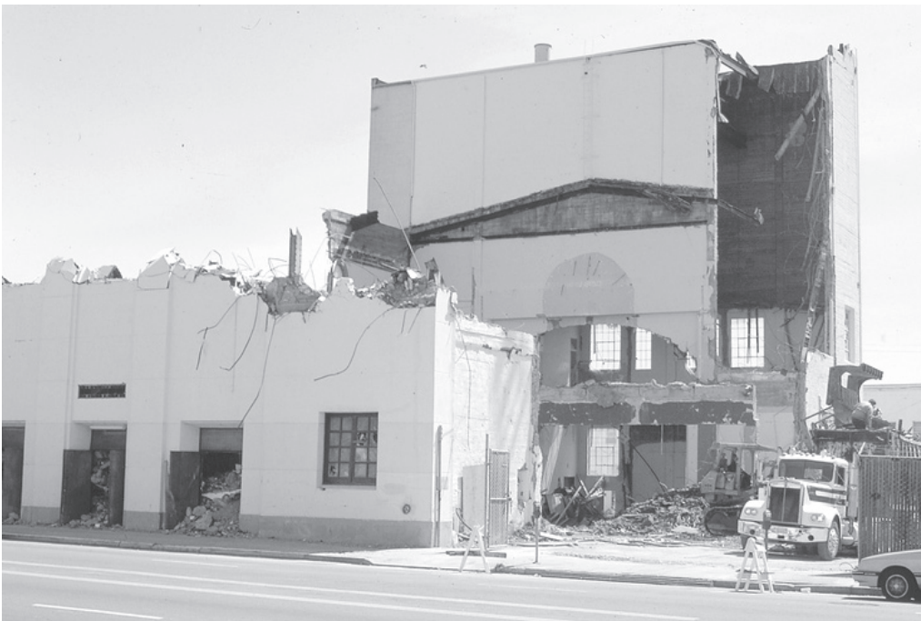
The Greek Orthodox Cathedral of the Annunciation being demolished after the 1989 Loma Prieta Earthquake. Max Kirkeberg Collection, DIVA, SF State.
