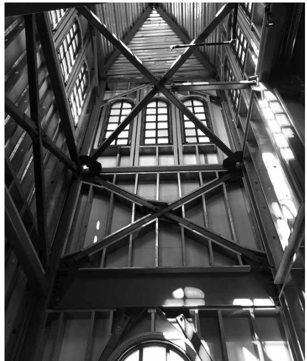
Looking up towards the "belfry," one is able to see the steel bones of our magnificent new Cathedral. Even though the interior currently lacks finished walls, one is inspired by the sheer height and proportions of the interior, ever lifting us up towards heaven, capturing the essence of what the Rus are said to have remarked upon entering the Great Church in Constantinople, a thousand years ago, "We knew not whether we were in heaven or on earth..."
