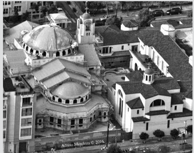
We've come a long way since the roof membrane went up, "back" in 2016. Since then, the dome and half dome were covered with standing seam copper; the tile roofing was laid; and the vertical walls were covered in stucco. Yet, this is an amazing photograph, taken high above, showing the Cathedral complex in its entirety. A visually stunning photo. Photo by Adrain Mendoza.
