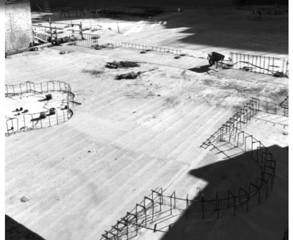
A view of the parking deck, upon which the vertical steel for the new Cathedral will be erected. (The parking component has already been completed, and lies below the deck.)
