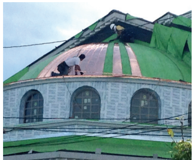
Copper being fitted over the ieron dome. The ieron dome will be clad following partial stucco of the area above it.
