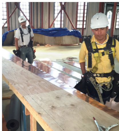
The copper is unrolled and made into strips for the domes or flashing. The gutters and downspouts are also being fabricated of copper.
