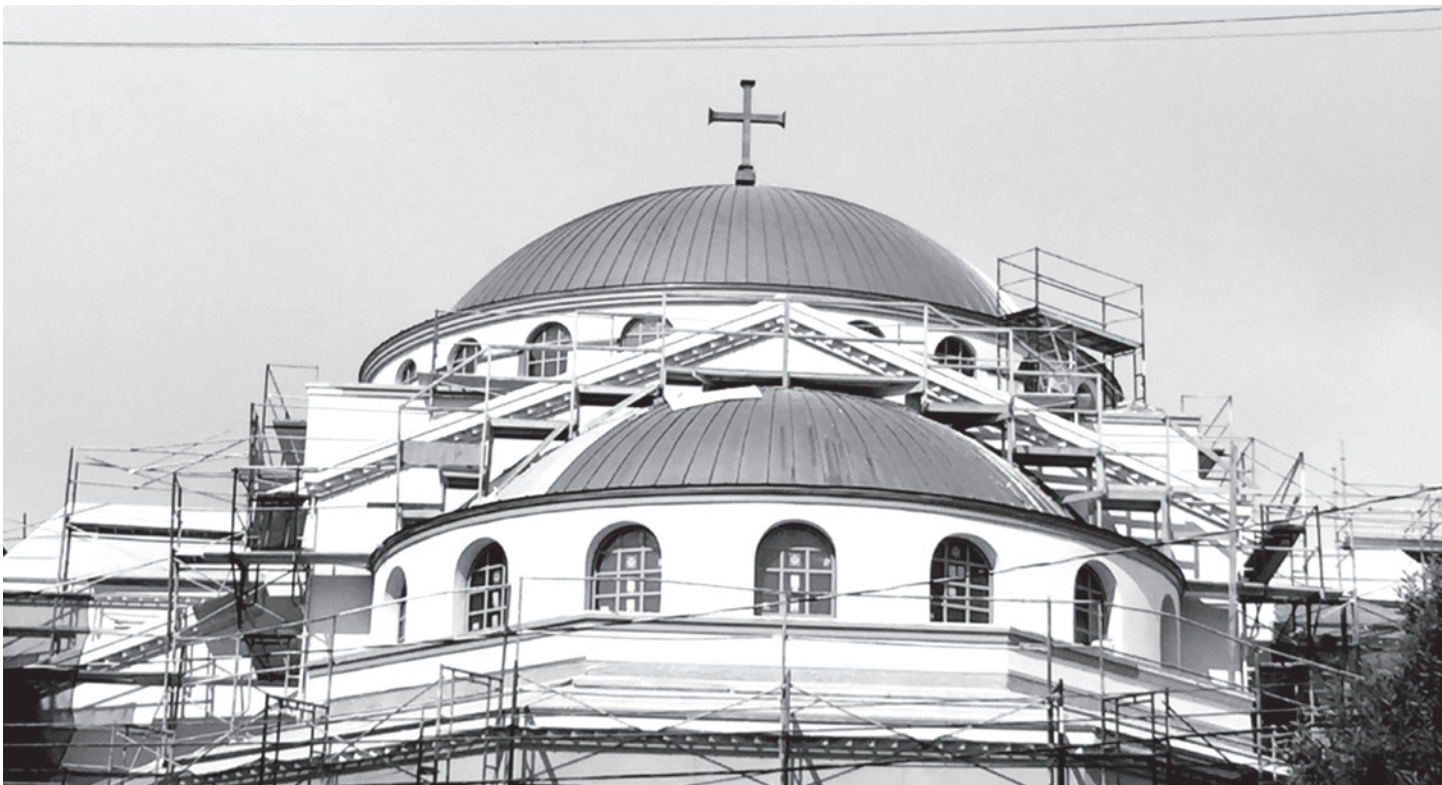
A view from Stevenson Street, behind the Cathedral, taken on the Feast of the Dormition (August 15), showing the massing of the ieron and central domes, the stucco work, the copper work, the painting, and the areas of the roof which will be covered with clay tiles during September.
