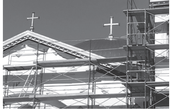
A partial view of the façade, showing the new crosses, prior to stucco.
