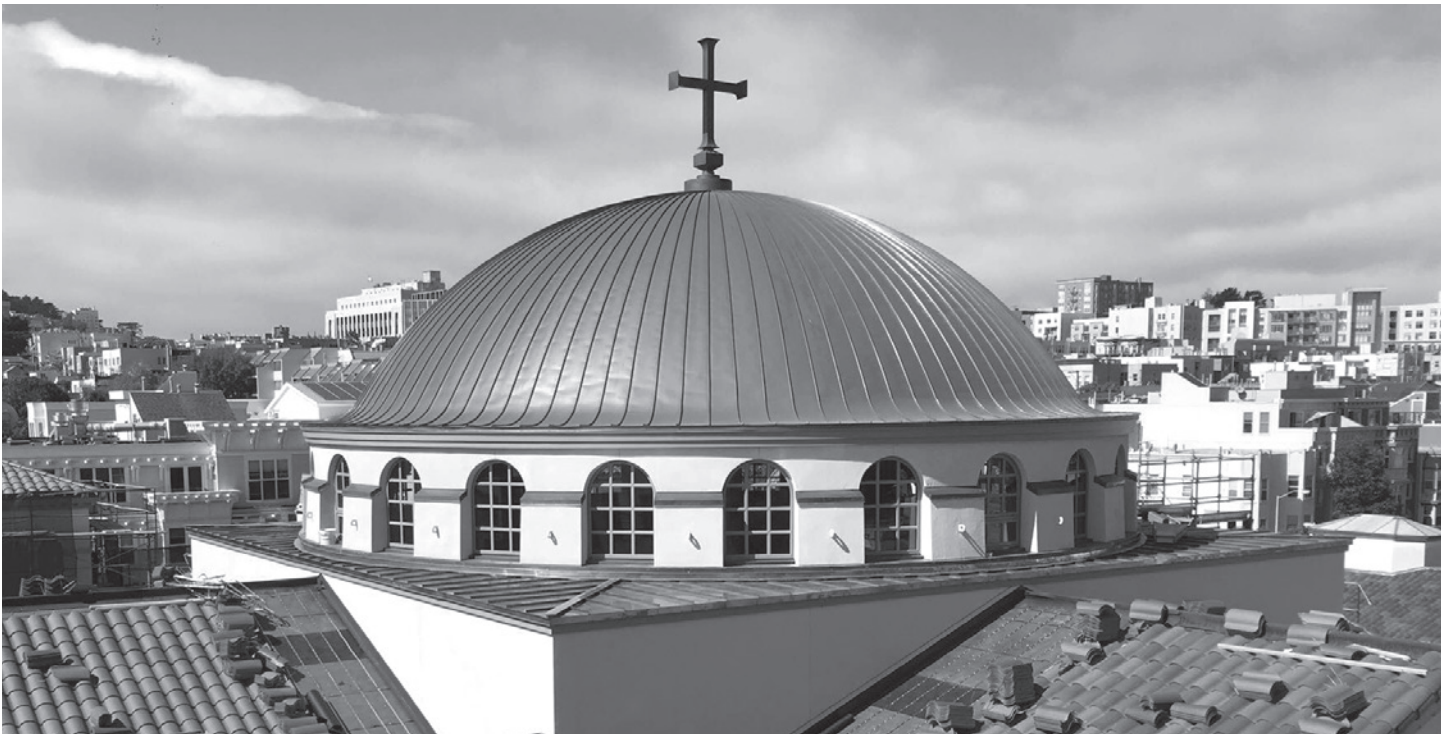
A magnificent view of the progress of the clay tile roofing being laid, the backdrop being the San Francisco skyline, looking northwest. Annunciation, literally, is in the heart of the City. The new Cathedral is shaping up to be the heart of the City.
